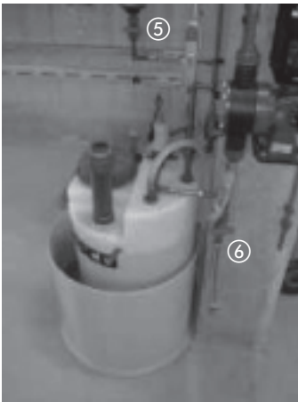
Fig. 6-4: Acidification tank with pump
